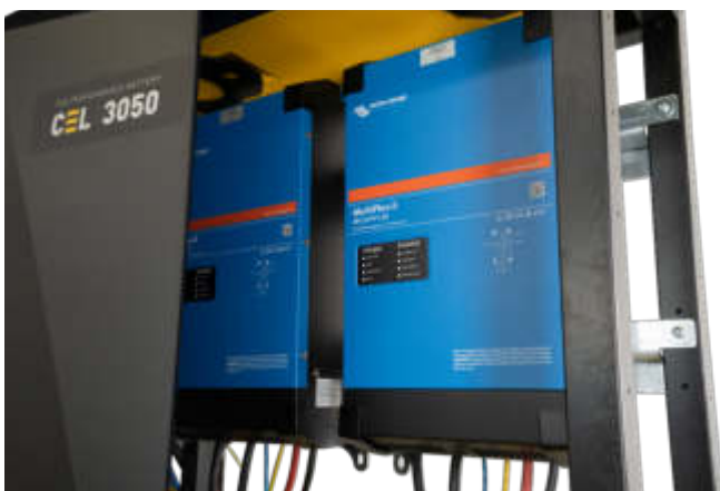
Interior view Cel-3050 10 kWh three-phase
